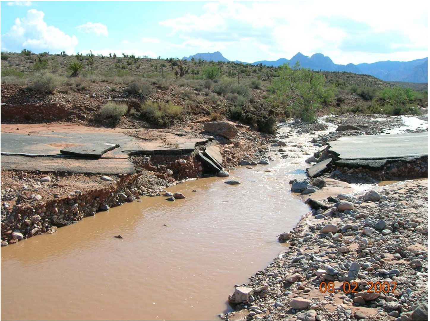
Damages to Calico Basin Road resulting from storm runoff on August 2, 2007.
