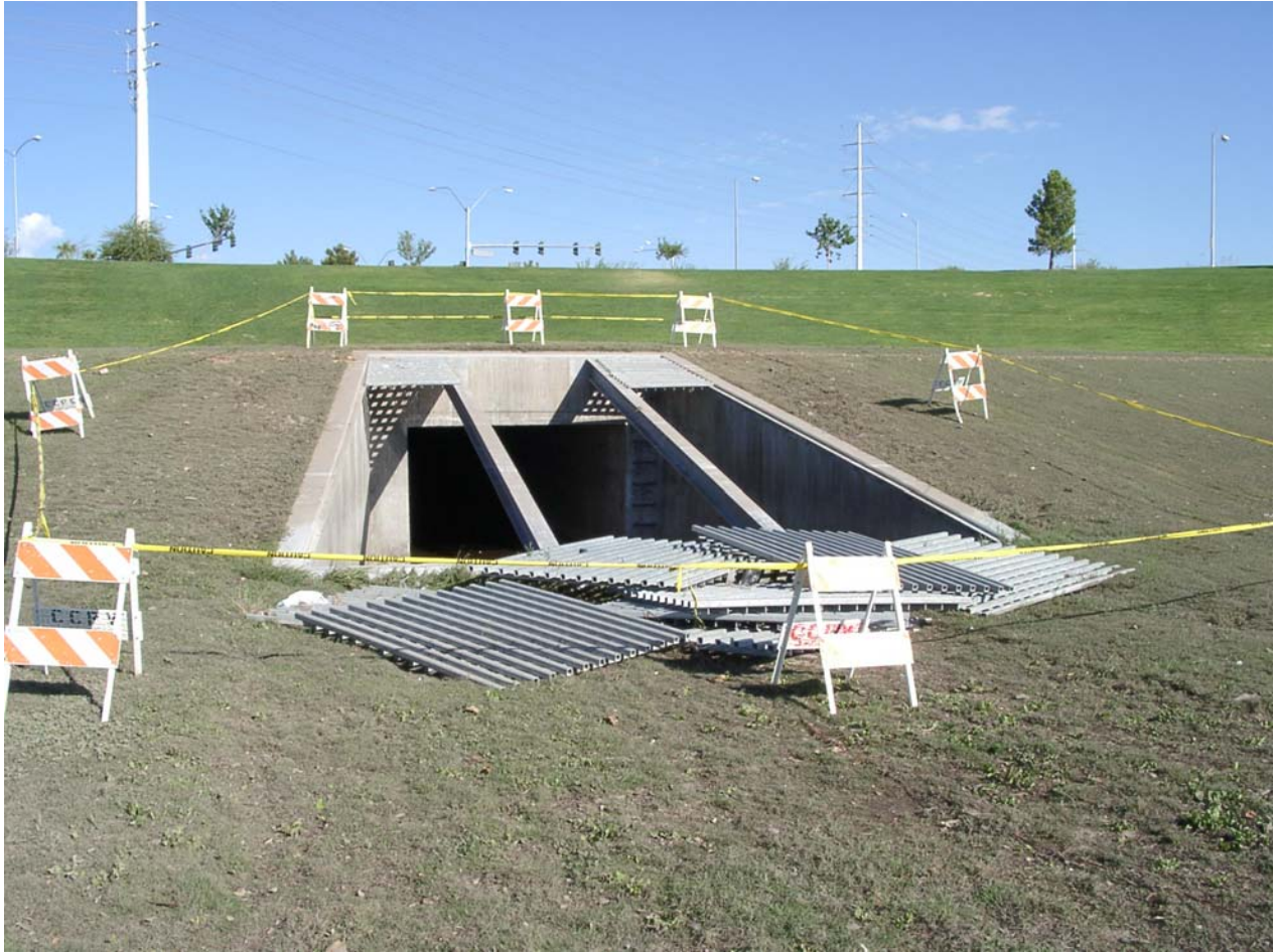
Figure 2. Grates covering inlet structure at northwest corner of The Lakes Detention Basin dislodged by flow entering the basin.
