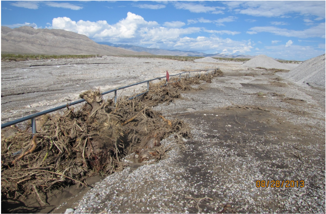
Figure 9. Northernmost inlet structure at Kyle Canyon DB, resulting from August 25, 2013 flooding
