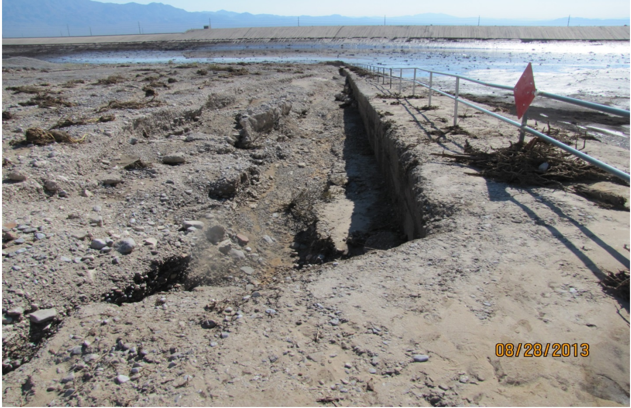
Figure 10. Erosion along inlet structure at Kyle Canyon DB, resulting from August 25, 2013 flooding
