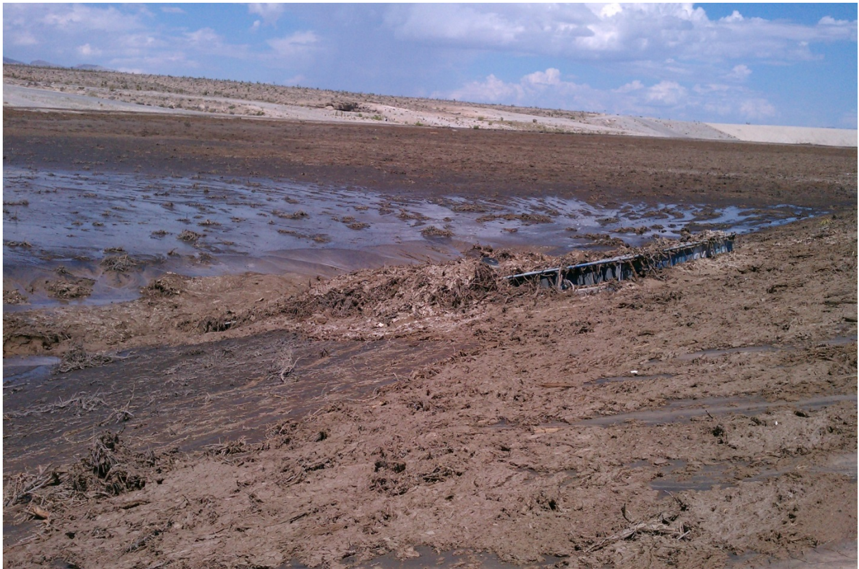
Figure 6. Debris washed into Kyle Canyon Detention Basin (August 28, 2013)
