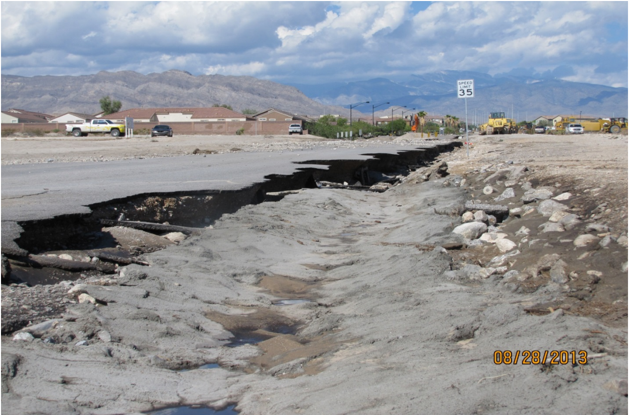
Figure 8. Damage to Grand Teton Drive resulting from August 25, 2013 flooding
